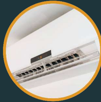
Air Conditioner tiap lantai
